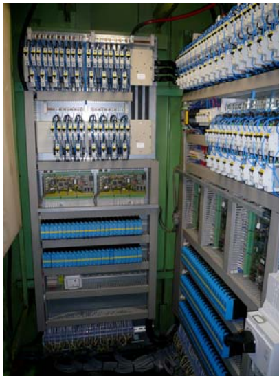
(3: new temperature control system ETC-24)
